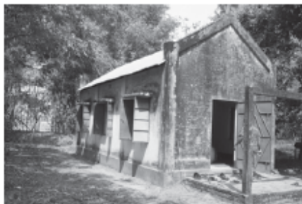
Nalkura church building shows its need for repair
